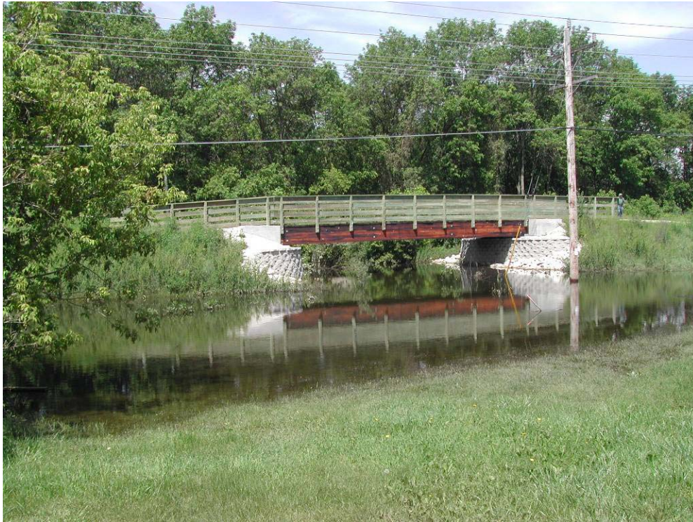
Pedestrian bridge along bike path on the west side of Main Street
