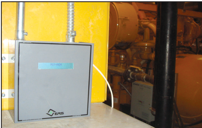
▲ The Monitoring & Control Server manages the collection and flow of data gathered from sensors in a building's utilities infrastructure.
