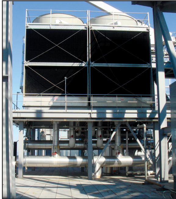
▲ A cooling tower atop a Manhattan office building is just one piece of the power and utilities equation being monitored by Embedded’s technology.
