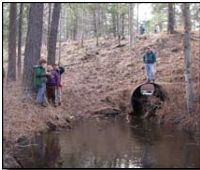
Researchers conduct a preliminary site assessment of an aquatic organism passage barrier on the Deschutes National Forest in Oregon.
