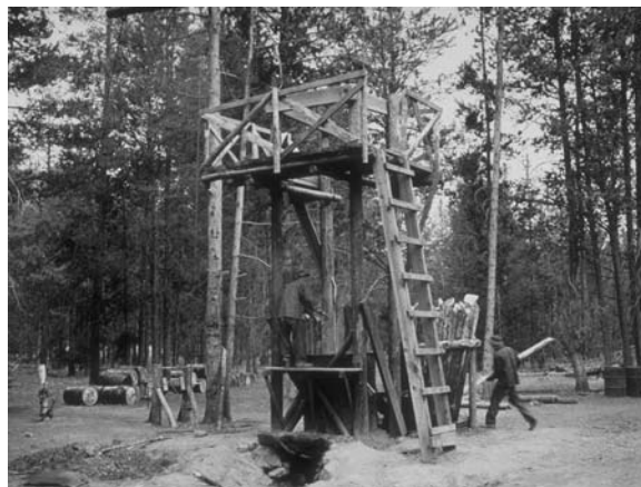
CCC enrollees preparing fence posts and telephone poles and operating creosote plant at Stewart Flat, 1941.
