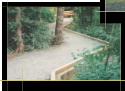
Simple timber retaining walls were used to wind this trail through the woods. Spirit Lake Memorial Highway, WA
