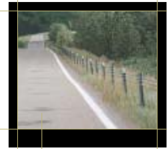
Cable guardrails are unobtrusive in this rural setting. Glacier National Park, MT
