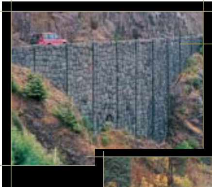
Using native stone to face this massive retaining wall makes it less visible from other sections of the road and blends with stone work used on the adjacent viewpoint. Pacific Coast Scenic Byway, OR
