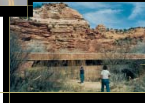
This bridge was textured and colored to be aesthetically pleasing to hikers who pass under it. Highway 12 Scenic Byway, UT
