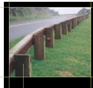
Steel-backed wooden guardrails are used to replicate the look of historic guardrails. Blue Ridge Parkway, VA
