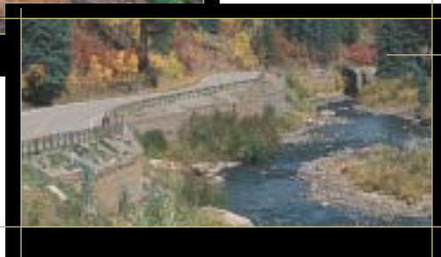
This welded-wire retaining wall along the West Delores Road was chosen because the color of the stone blends into the environment, and it was less expensive than a concrete wall. San Juan National Forest, CO
