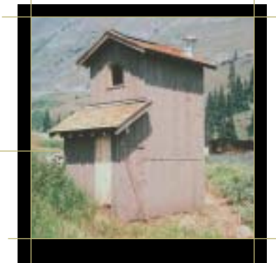
Built to reflect the mining history of the area, this Bureau of Land Management composting toilet fits comfortably in its surroundings. Alpine Loop National Back Country Byway, CO
