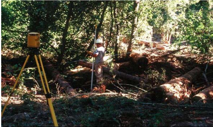
Figure 8. Among other things, field crews measured the shape of the floodplain and stream channel at 24 sites within the treatment reach. This information will help document and describe stream channel shifts resulting from large wood placement.
