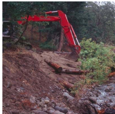
Figure 4. At many sites, logs were placed in and along stream banks not only to reduce erosion but also to prevent the stream from shifting into the new trail. At these locations, the excavator was often able to work from the bank to place and bury logs.
