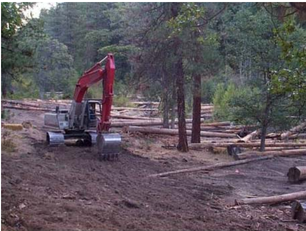
Figure 5. This section of road was completely removed from the landscape by digging it up and restoring the natural contour of the land. We spread native grass seed and straw mulch and now the area is covered with grass.
