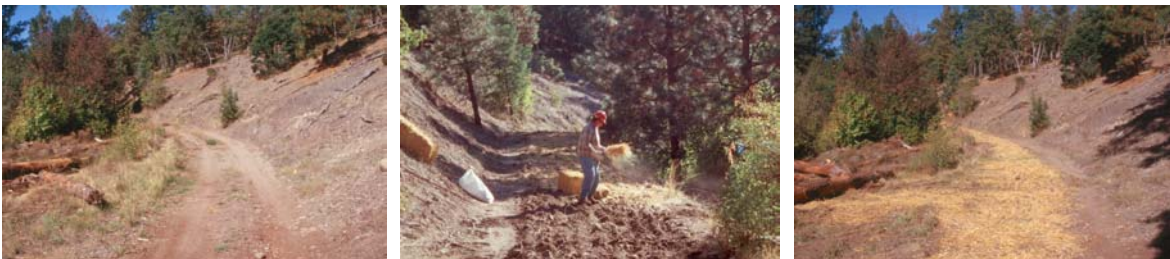
Figure 6. Example of a section where the road was sloped away from the hillside, scarified except for the trail area, seeded with native grass seed, and mulched. The left and right photographs are before and after photos of the same location.
