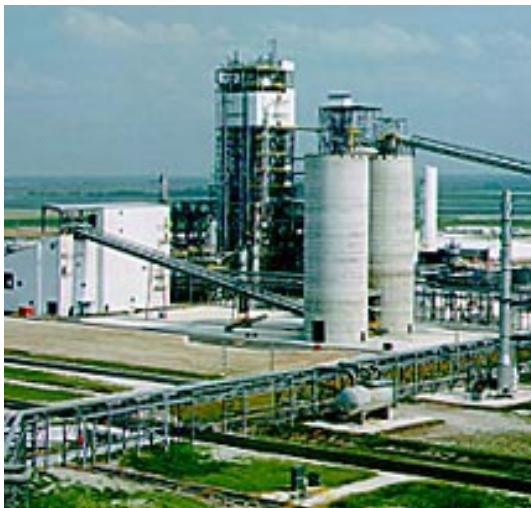
The Tampa Electric Company's pioneering gasification combined cycle facility is one of the cleanest and most efficient coal-fired power plants in the world.
