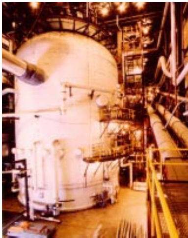
The 70-megawatt Tidd Pressurized Fluidized Bed Combustor pioneered a new, cleaner way to burn coal in utility power plants.
