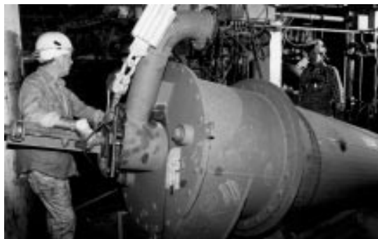
Technicians install an advanced low-NOx burner into a retrofitted boiler at Southern Company Services' Plant Hammond.
