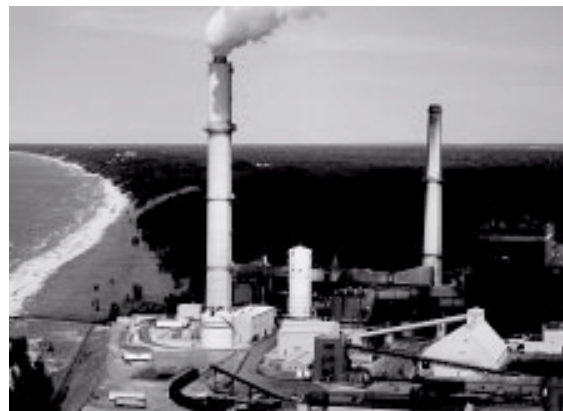
Equipped with the Pure Air advanced desulfurization unit, the Bailly Station on the shores of Lake Michigan is now removing more than 95 percent of the sulfur pollutants from its coal combustion flue gas.
