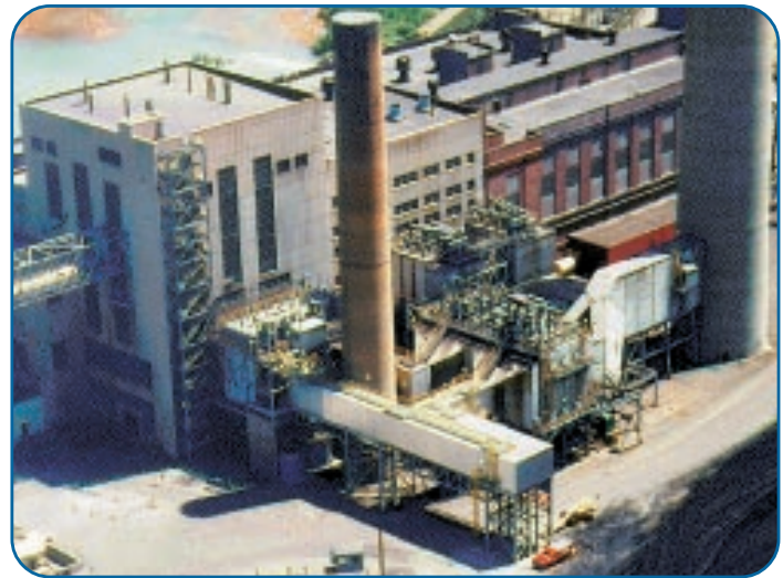
Bechtel CZD installation at Seward Station
