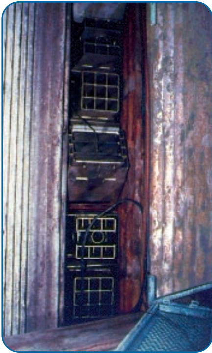
LNCFS™ Low-NO x Burner at Plant Lansing Smith
