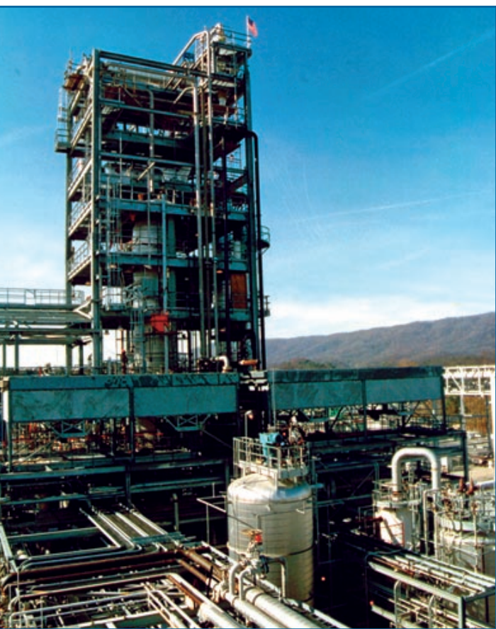
LPMEOH™ installation at Eastman Chemical Company
