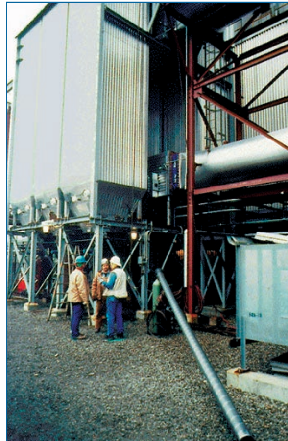
The SNRB™ appears in the background and the SCR catalyst holder in the foreground at the R.E. Burger Plant
