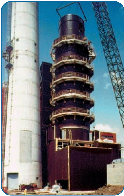
LIFAC installation at Whitewater Valley Station
