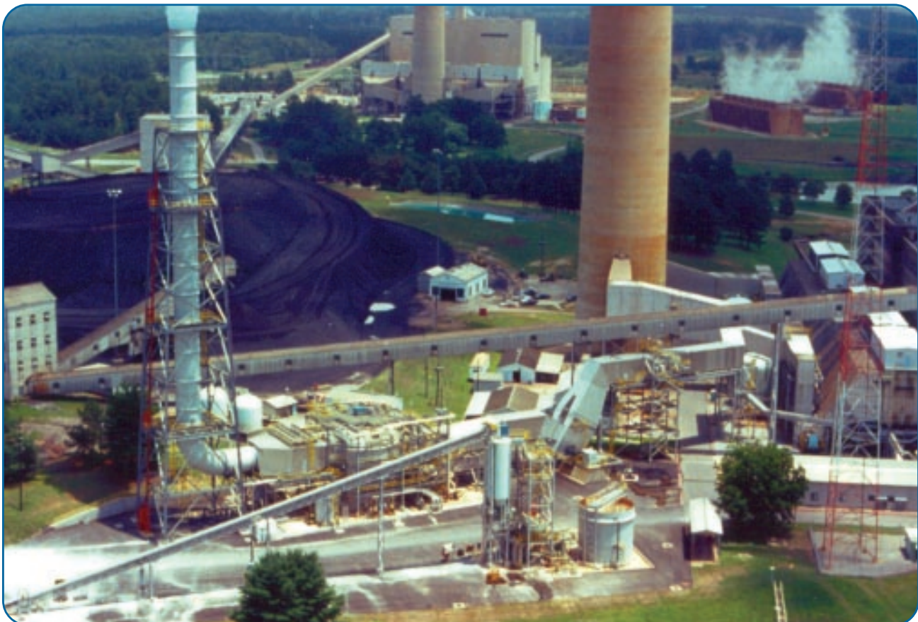
CT-121 installation at Plant Yates
