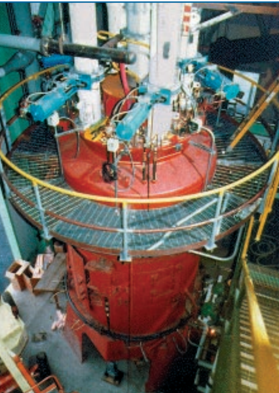
Coal pulverizer used to supply Babcock & Wilcox reburning system at Nelson Dewy Station
