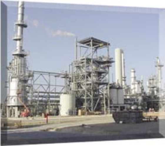
Operating since 2000, the Brisbane Hydrogen Plant in Australia employs two GE Energy gasifiers with natural gas as the feedstock to produce chemicals.
