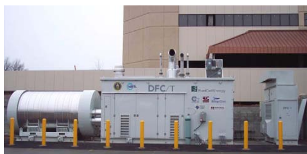
FIGURE 4. Alpha DFC/T ® Unit after Installation at Billings Clinic, the Montana Demonstration Site
