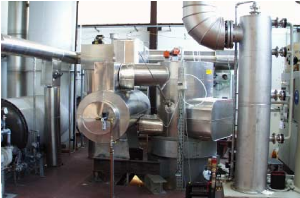
Fig. 3 View of the filter of the pyrolysis pilot plant at the Karlsruhe Research Centre
