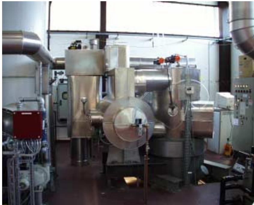
Figure 1: Pilot filter as a part of the pyrolysis plant “PYDRA” at the Research Center of Karlsruhe.
