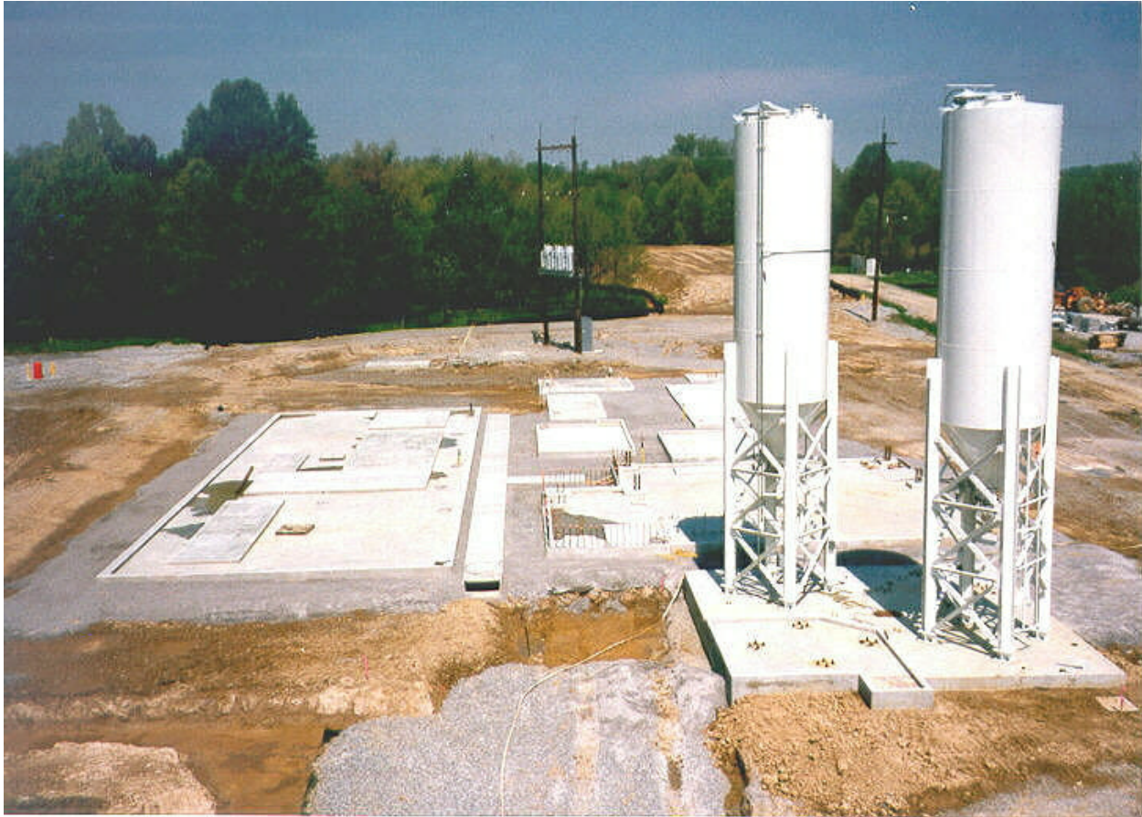
Figure 2 Photograph of Equipment Pads at Paducah Site
