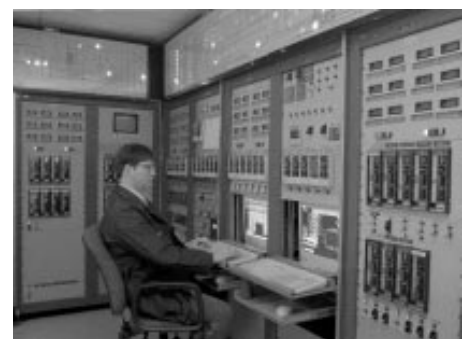
The Control Room for the Fluid-Bed Gasifier
