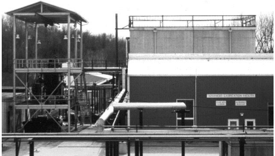
METC's Modular Gas Cleanup Rig (MGCR) , at left, and Fluid-Bed Gasifier , on the right, combined form the METC Gasification and Hot Gas Cleanup Facility .
