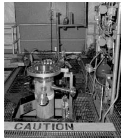
MGCR Particulate Removal and Desulfurization Equipment
