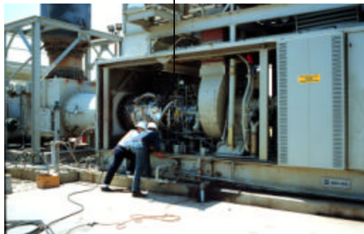
Centaur 50S Engine at Texaco Site
