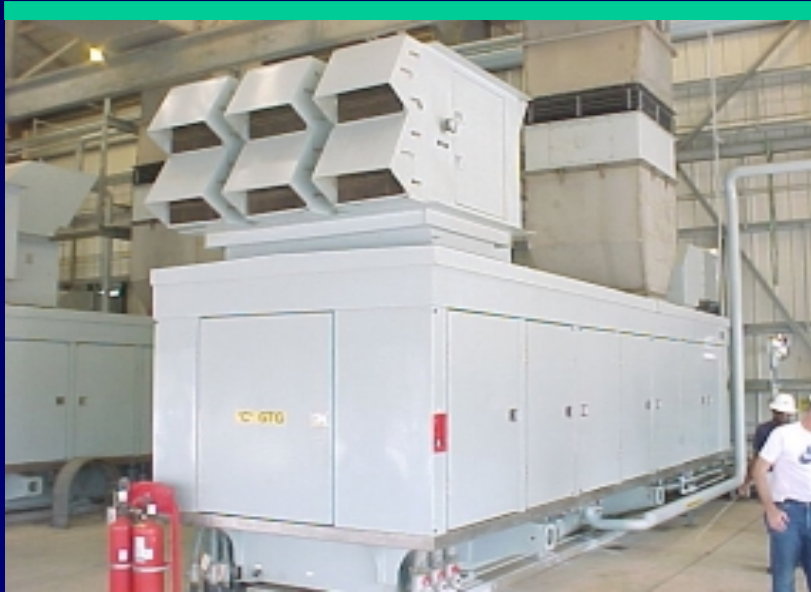
EXXON Natural Gas Processing Plant - Engine Skid
