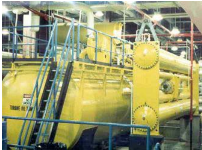
Figure C.10: Example of a Lube Oil Tank in Turbine Hall
