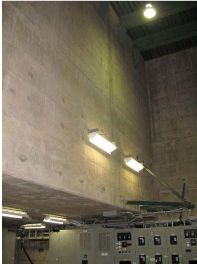
Figure B.2: Example of a Switchgear Room
