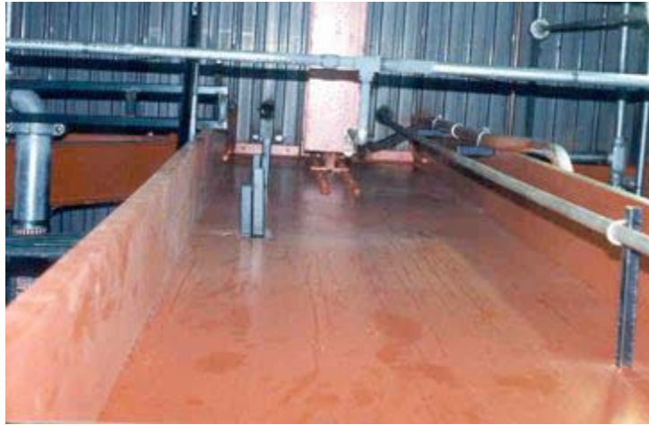
Figure C.5: View of Steel Beam Looking up at Ceiling Depicting Beam Sprinklers
