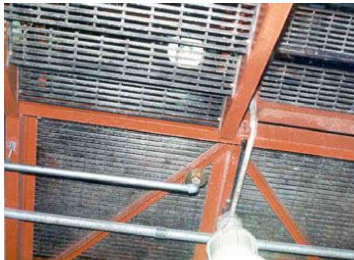
Figure C.6: Example of the Open-Grate Stairs and Walkway with Sprinkler Underneath
