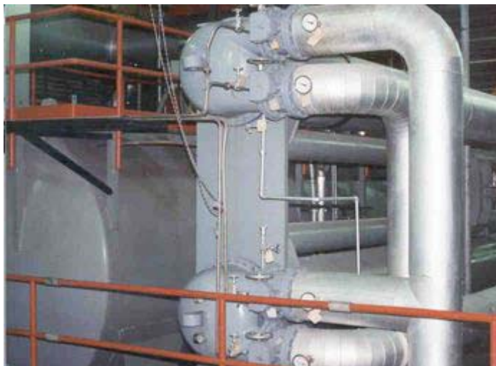
Figure C.11: Second Example of a Lube Oil Tank in Turbine Hall
