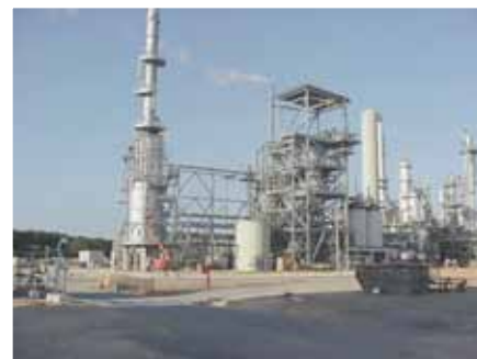
The Brisbane H 2 Plant in Australia has been operating since 2000 and employs two GE Energy gasifiers with natural gas as the feedstock to produce chemicals.
