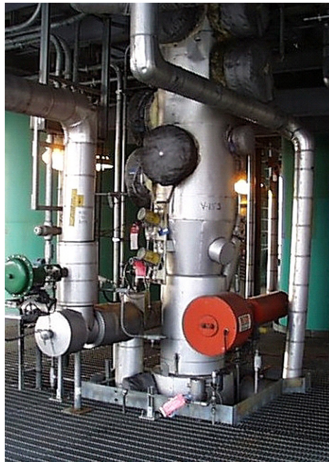
Filter vessel installed at Wabash plant
