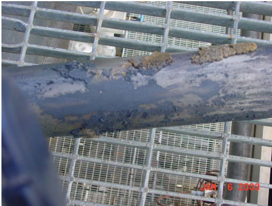
Figure 4.3-17 Back-Pulse Pipe After TC10
