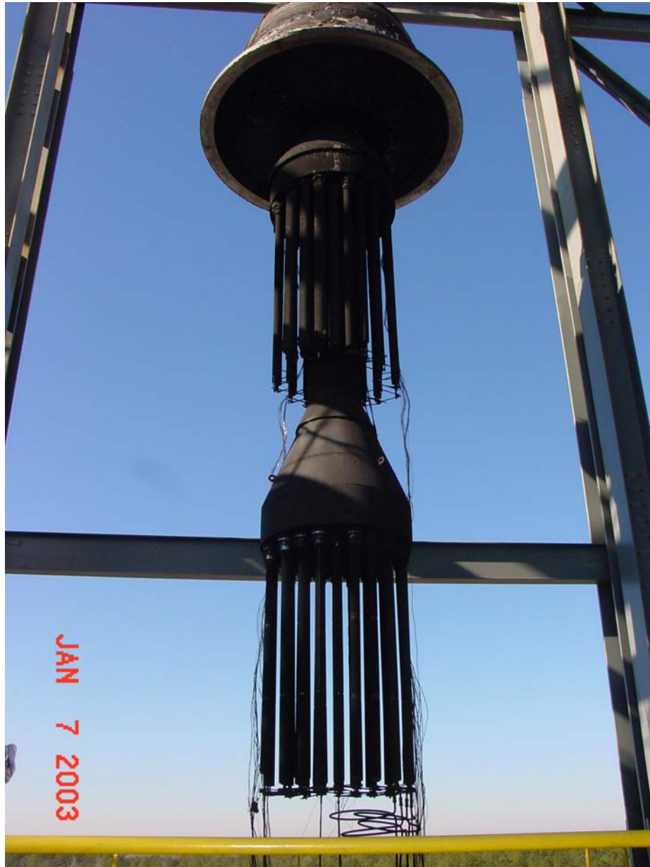
Figure 4.3-1 Filter Internals After TC10
