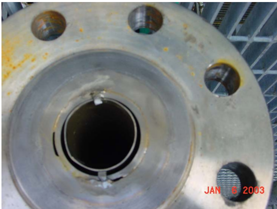
Figure 4.3-18 Back-Pulse Pipe Inner Liner After TC10
