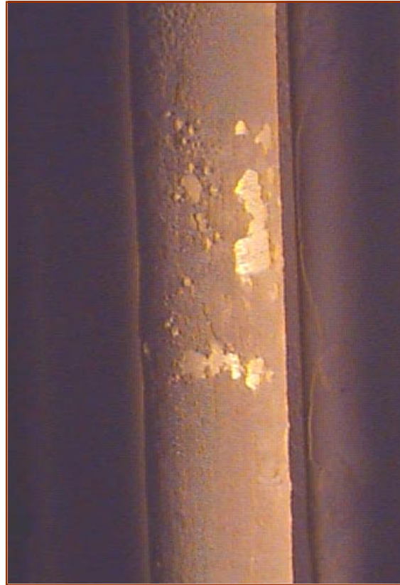
Figure 3.3-8 Possible Leaks on Techniweave Composite Filter Element (T17)
