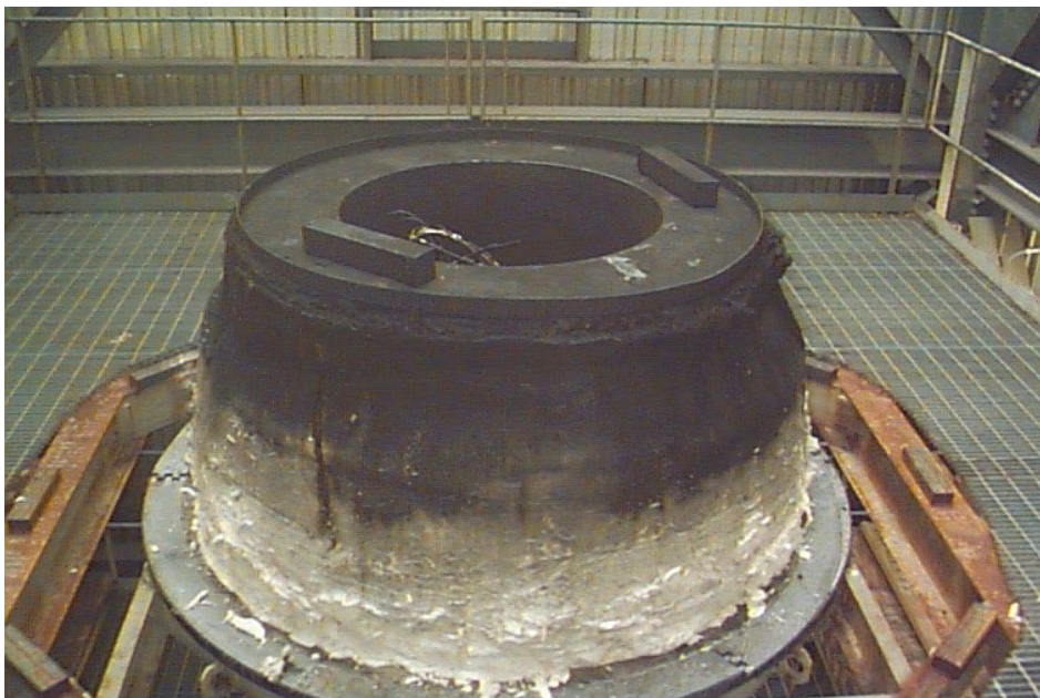
Figure 3.3-22 Tubesheet Insulation (GCT1B Through D)
