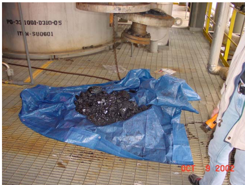
Figure 4.1-10 Tar Removed From HX0402 Gas Exit
