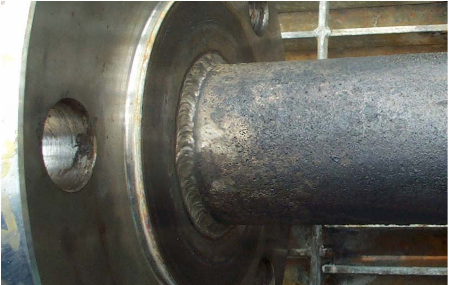
Figure 3.3-13 Pitting on Back-Pulse Pipes After TC08
