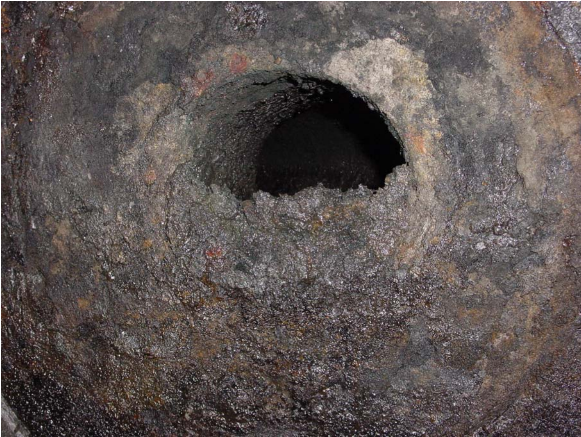
Figure 3.3-15 Material Found During Outlet Duct Inspection
