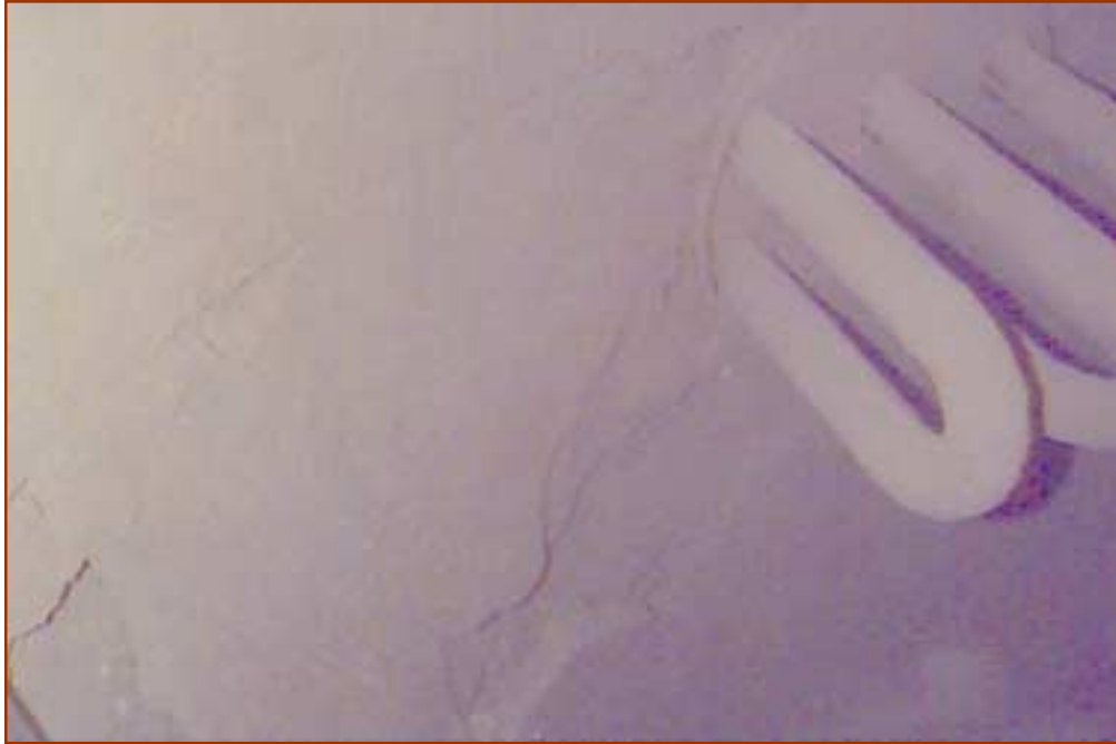
Figure 4.6-1 Sulfator Refractory Damage Following GCT2
