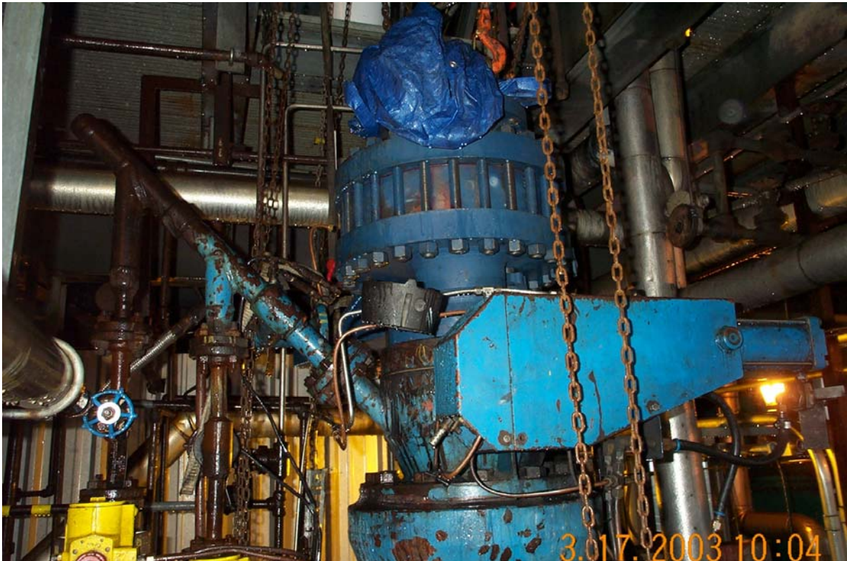
Figure 4.3-15 Everlasting Valve Installed Before TC11
