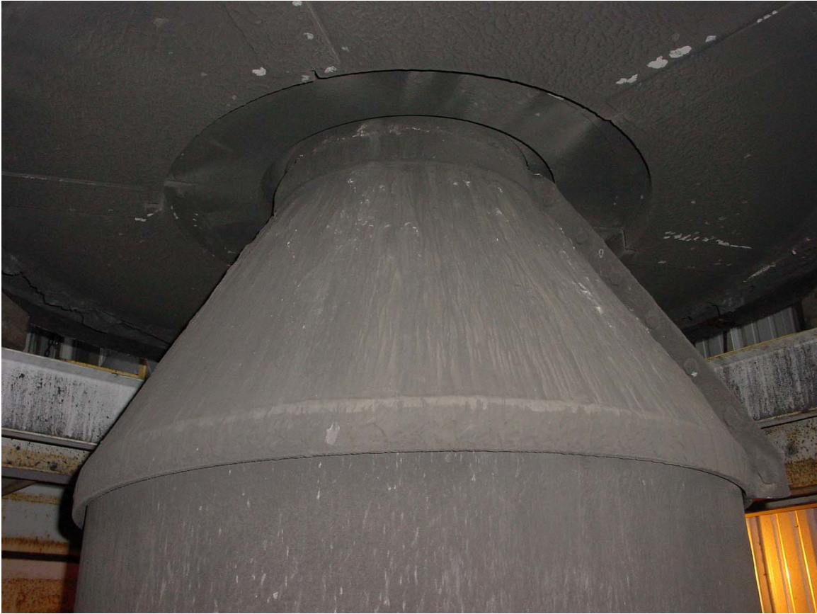
Figure 3.3-14 G-ash Build-Up on Upper Ash Shed After TC07D
