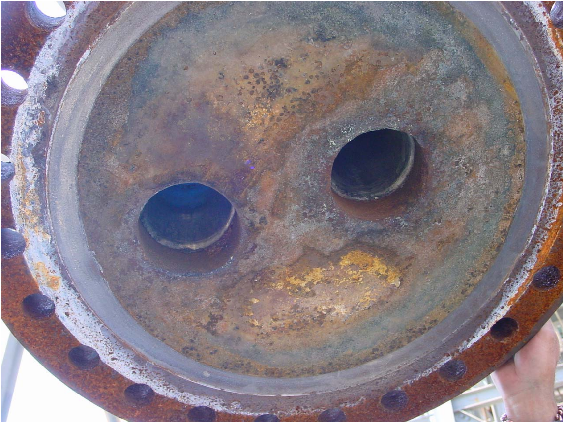
Figure 3.3-29 Nozzle 13 Flange After TC07D
