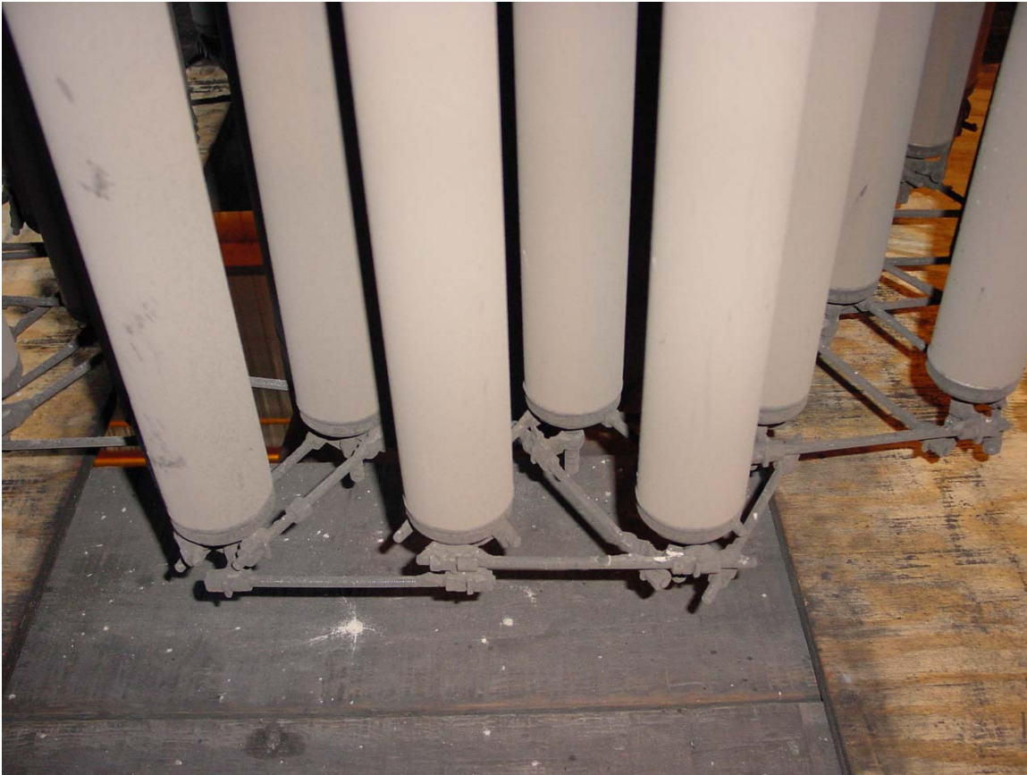
Figure 3.3-15 G-ash Build-Up on Support Brackets After TC07D
