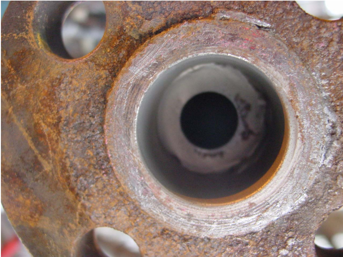
Figure 3.3-33 FD0520 Vent-Line Flange
