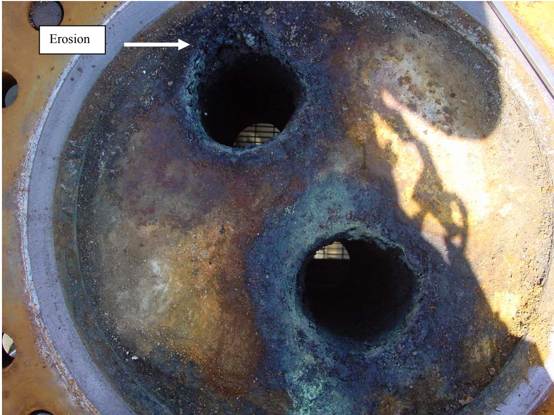
Figure 3.3-30 Nozzle 13 Refractory Erosion
