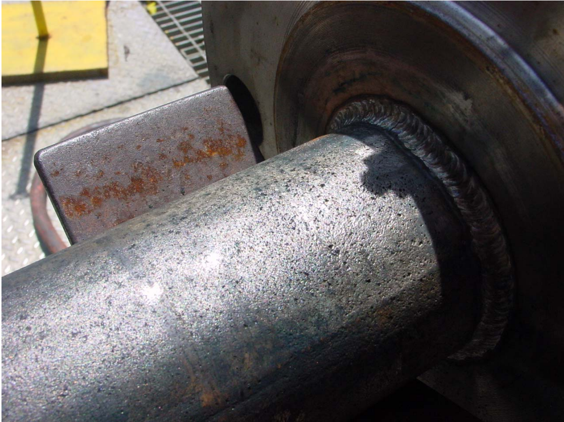
Figure 3.3-28 Pitting on Back-Pulse Pipe After TC07D
