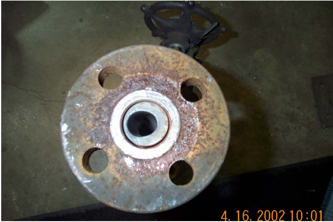
Figure 3.3-32 Erosion of FD0520 Vent Line After TC07D
