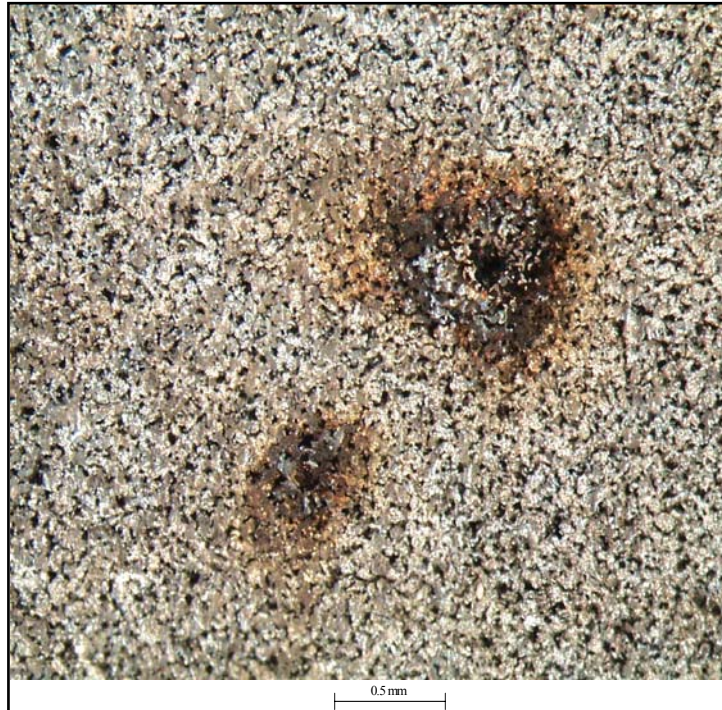
Figure 3.3-8 Pitting on the Outside Surface of Pall \text{Fe}_3\text{Al} Element 27060 Removed From Plenum Location B-35 After GCT4
