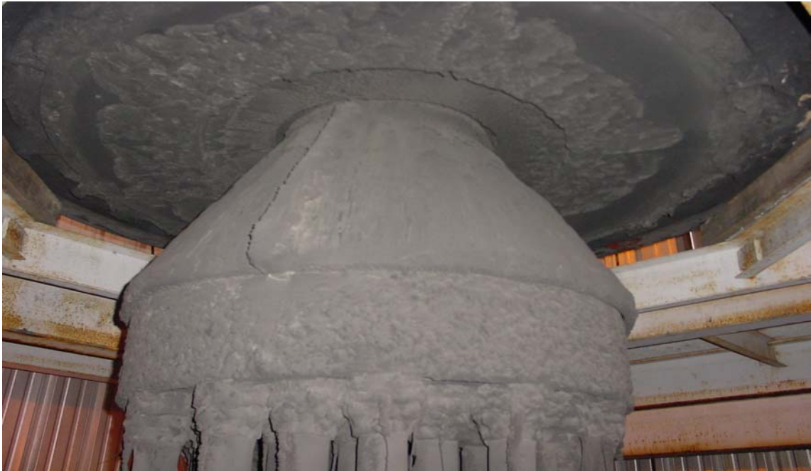
Figure 3.3-3 Char Build-up on FL0301 Top Plenum Surfaces
