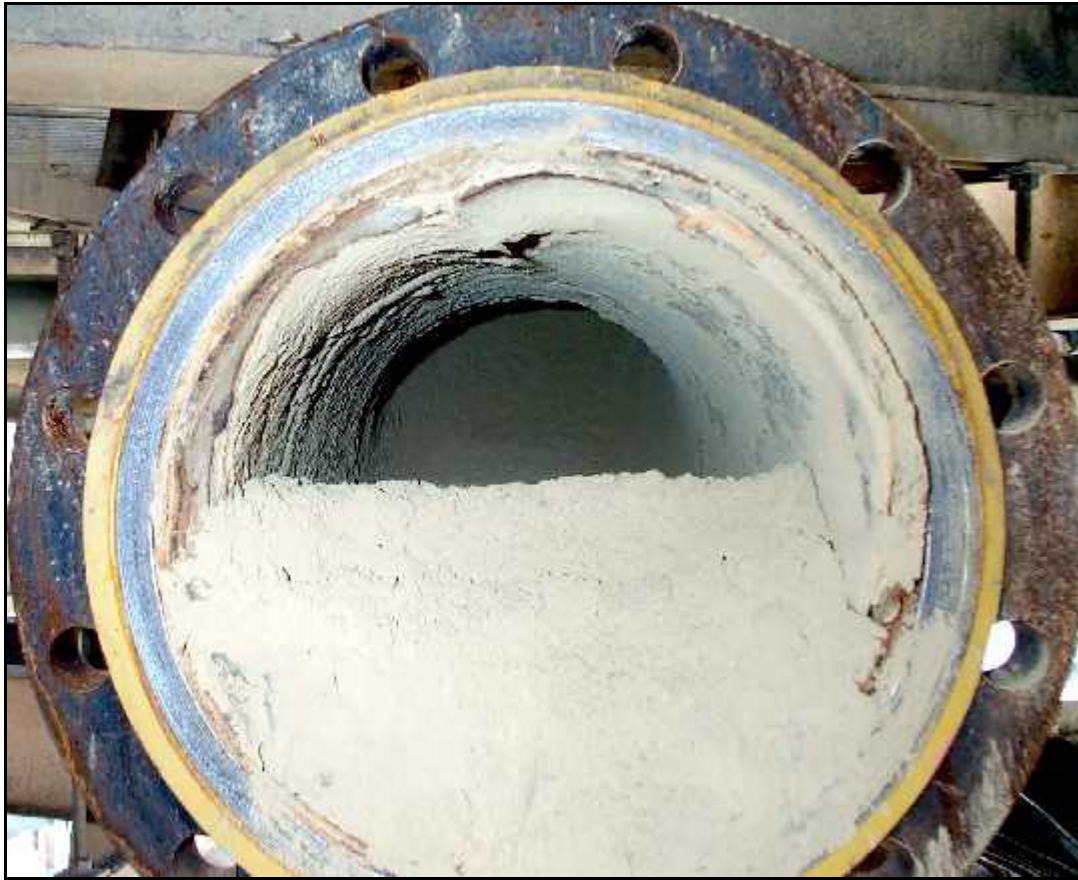
Figure 4.6-1 Solids Salted in Sulfator Flue Gas Line
