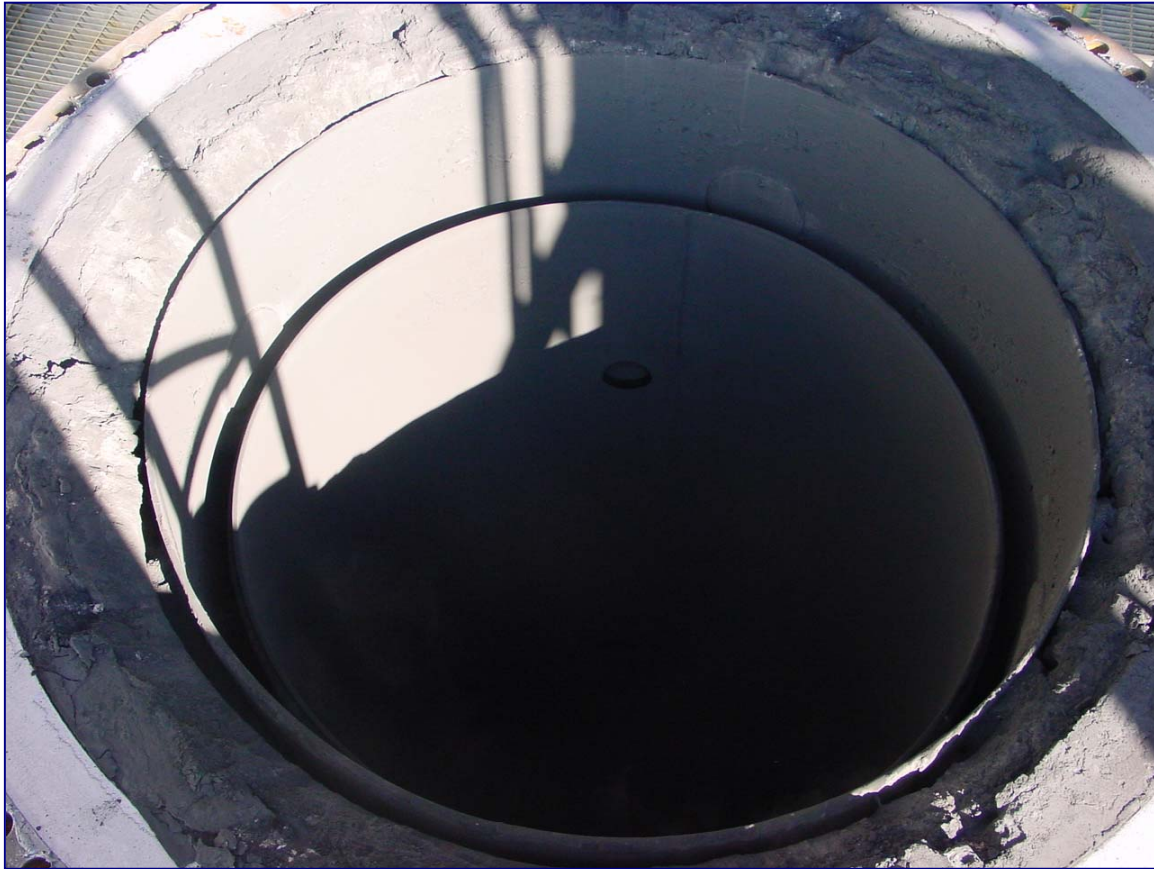
Figure 3.3-7 Char Accumulation on Shroud and Liner Section
