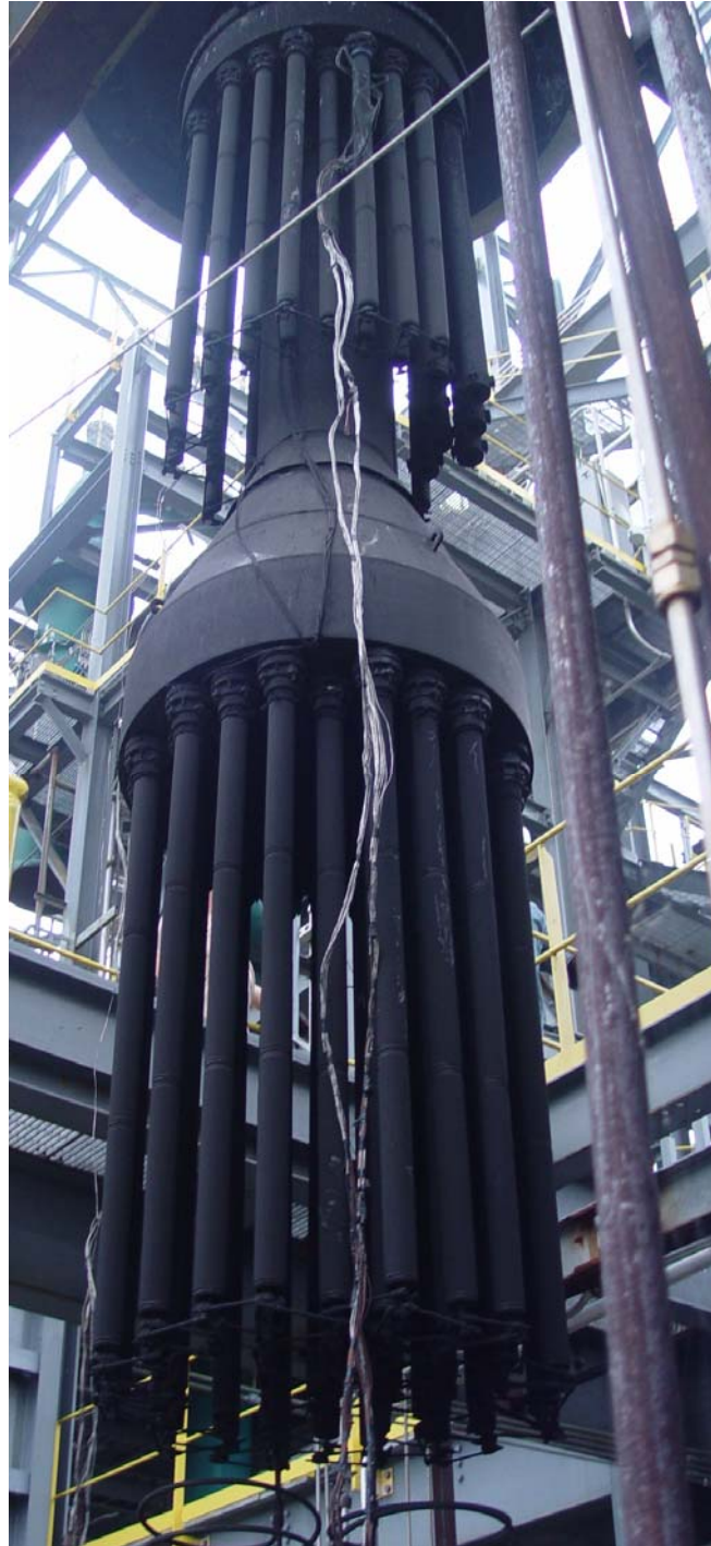
Figure 4.3-9 Filter Internals After TC13
