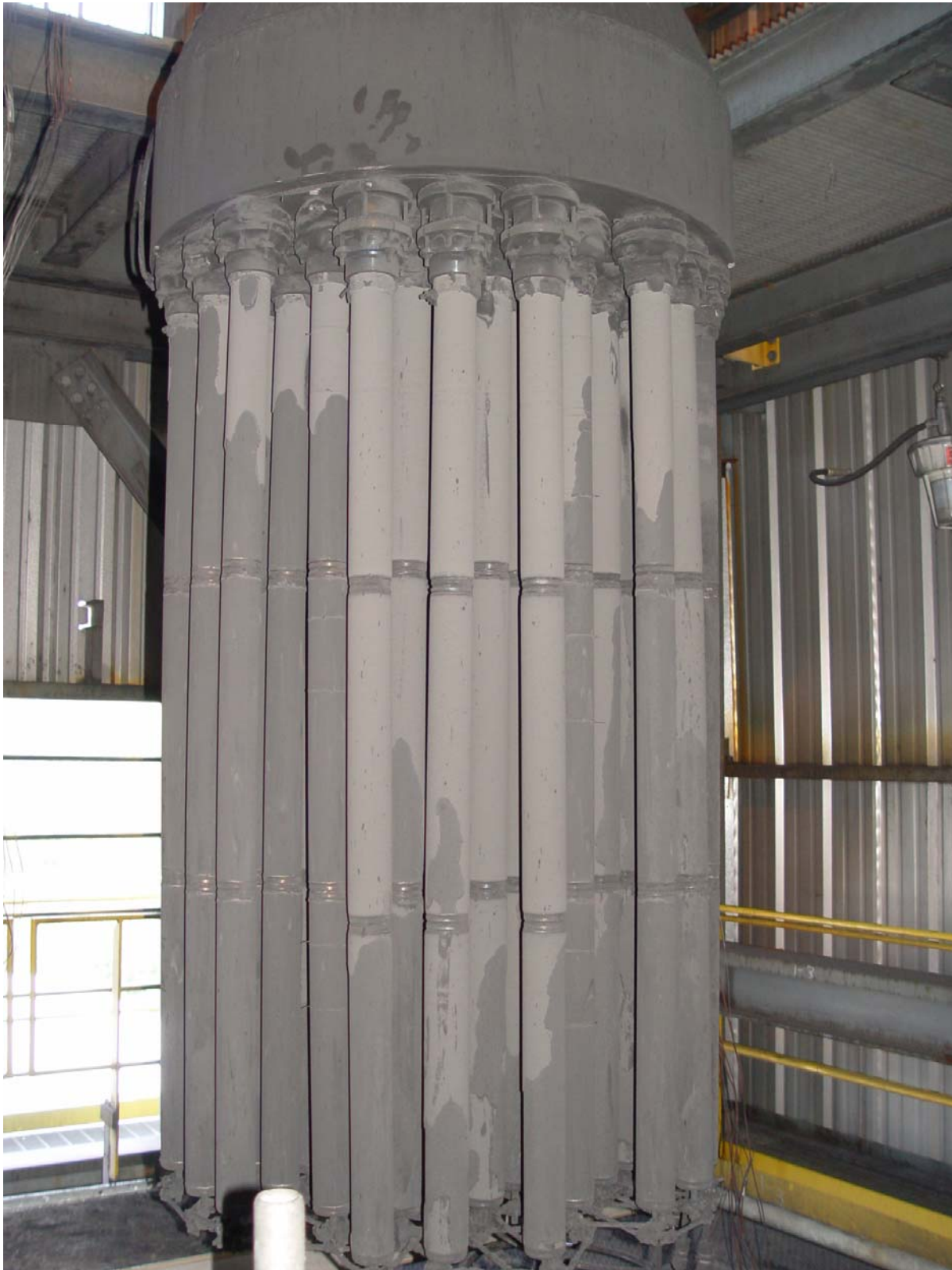
Figure 4.3-3 Bottom Plenum After TC12
