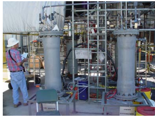
Figure 10. Solution Scrubbers in Syngas Cleanup Facility.
