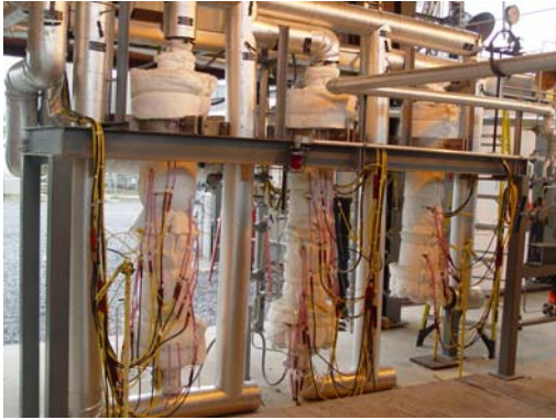
Figure 9. Small Reactors in Syngas Cleanup Facility.
