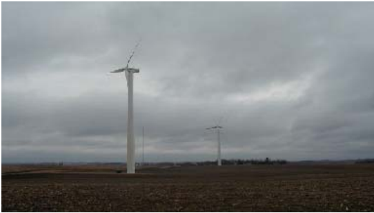
Large Wind Energy Conversion Systems
