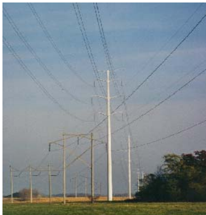
High Voltage Transmission Lines
