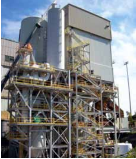
CFBDS and Baghouse
