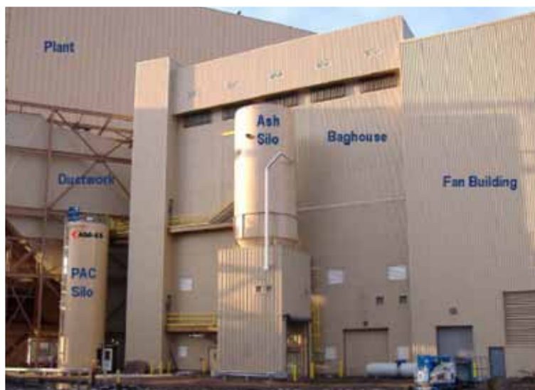
TOXECON® System Installed at PIPP
