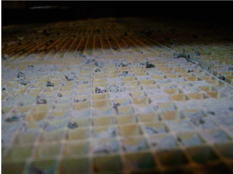
Figure 3. Photograph of a portion of the SCR catalyst (inlet end) taken during the December 2007 outage. Small pieces of LPA can be seen protruding from some of the catalyst channels.
