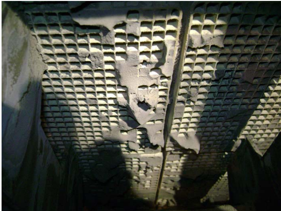
Figure 5. Photograph of a portion of the outlet end of the SCR catalyst taken during the December 2007 outage. Weak agglomerates of fly ash can be seen protruding from some of the catalyst channels.
