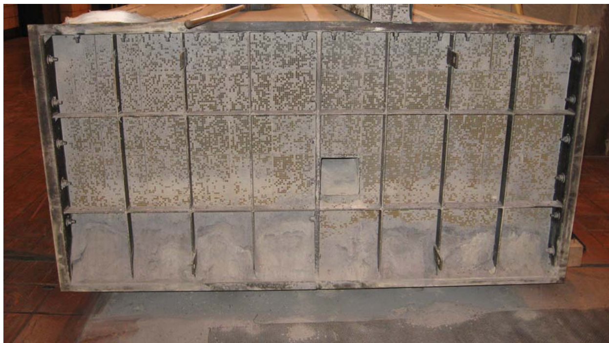
Figure 2. Photograph of a partially plugged catalyst module (viewed from the inlet end) that was removed from the in-duct SCR reactor during the late December outage.
