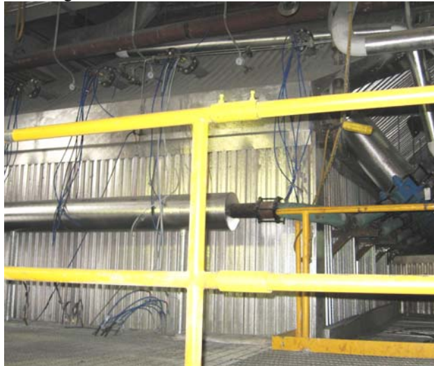
Figure 2. Photograph of the in-duct SCR reactor at AES Greenidge Unit 4.
