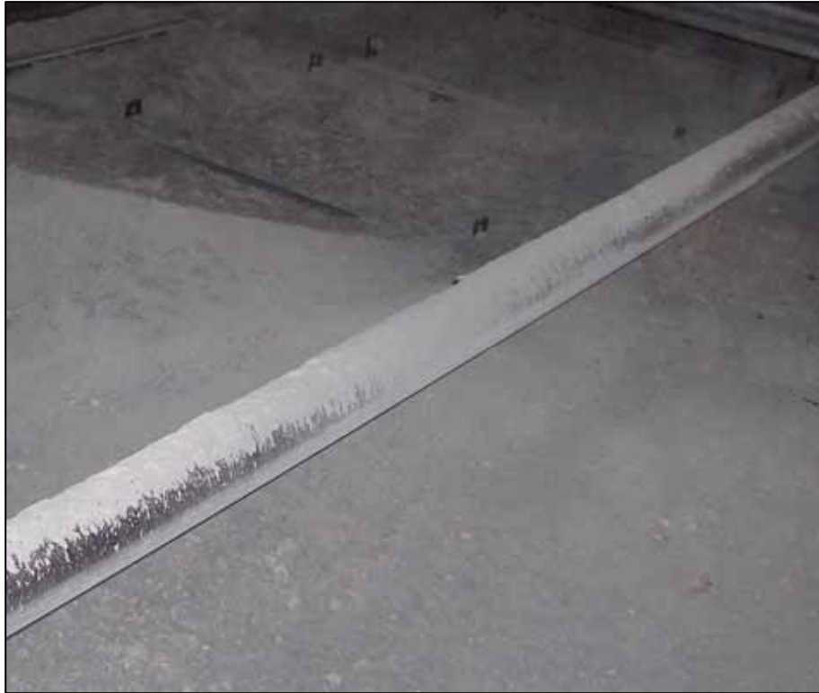
Figure 3. Photograph taken on February 3, 2007, showing the accumulation of large particle ash on the surface of the in-duct SCR catalyst.
