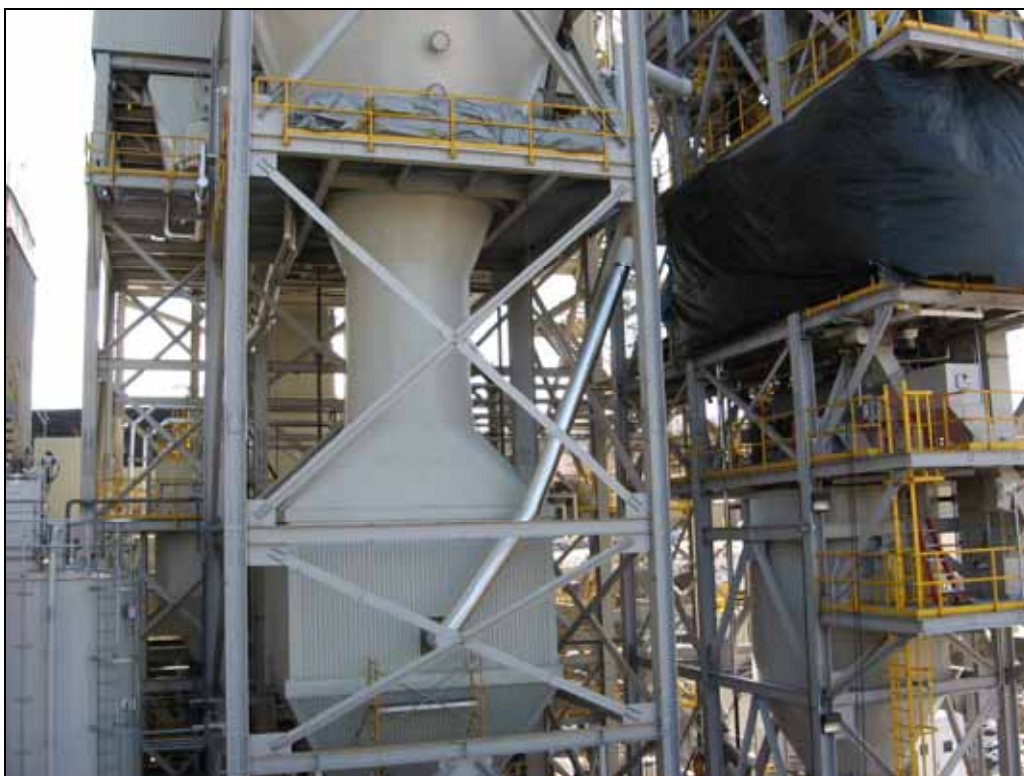
Figure 2. Photograph showing the installation of the new ductwork used to transport the hydrator exhaust to the inlet of the Turbosorp ® vessel.
