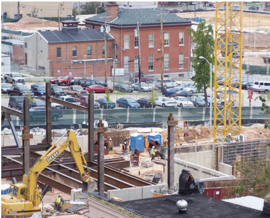
Tearing down buildings without tearing down health. Concerns about environmental hazards of demolition, such as debris left on sidewalks (top), were documented by the Environmental Justice Partnership Community Board, resulting in a set of safer practices that have been used in projects such as those by East Baltimore Development, Inc. (bottom).
