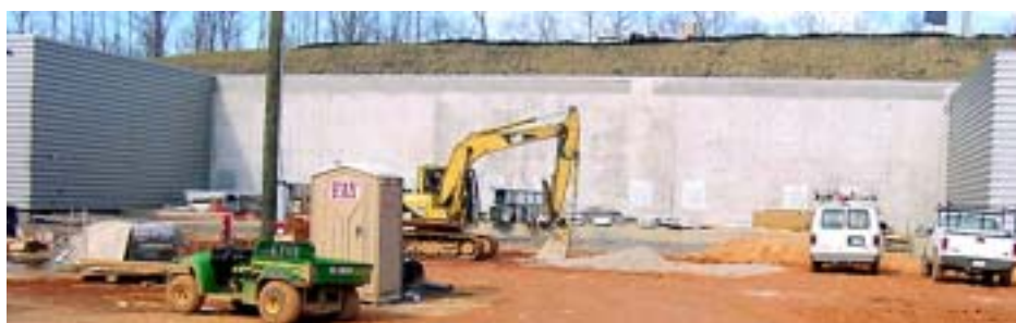
SNS Power Upgrade: The linac tunnel is sized for 9 additional “cryomodules” (top). Augmenting Klystron Gallery is required (bottom).
