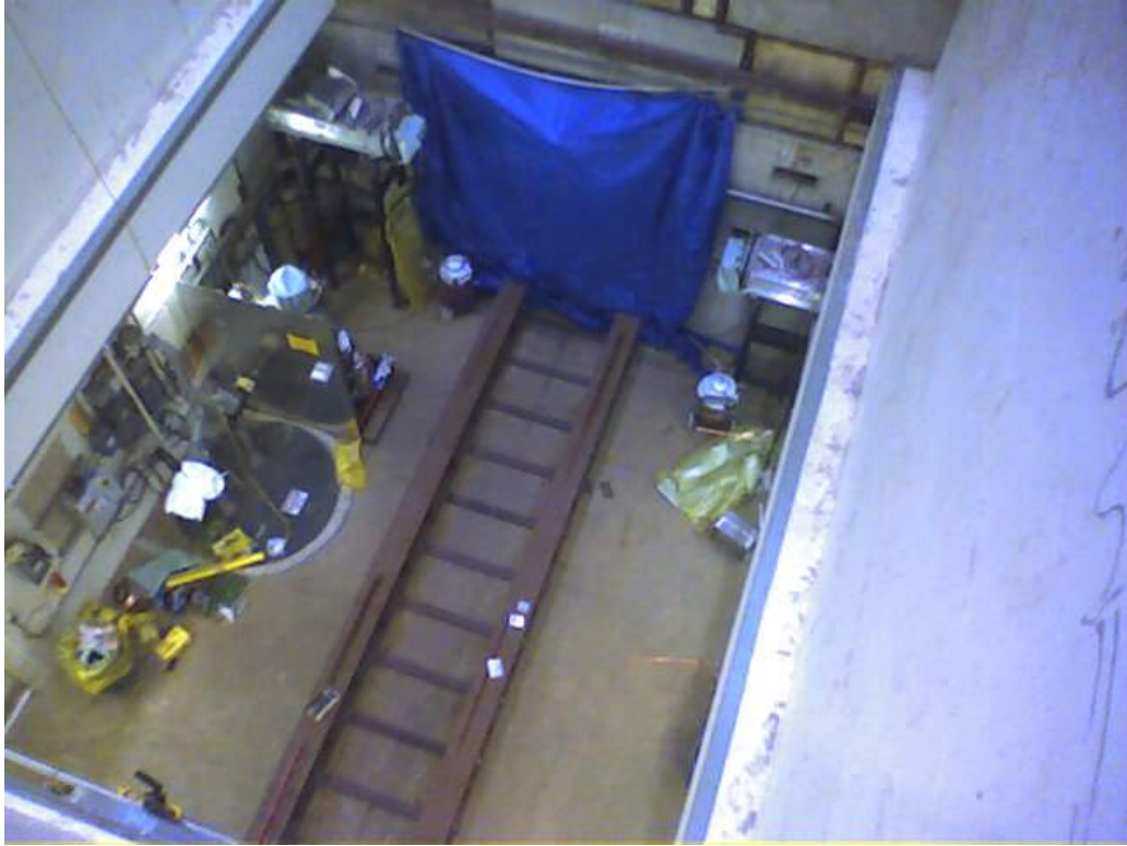
Blue Curtain Pulled Down Over Air Barrier in MI-12 B Enclosure Before Horn Removal
