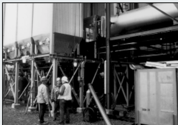
Bottom of baghouse where ash is removed and sent to storage silo with catalyst holder tube in foreground.
