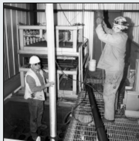
Workers lower one of the catalyst holder tubes into a mounting plate in the penthouse of the high-temperature baghouse.
