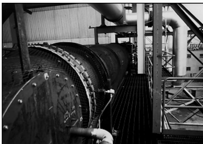
Lime sorbent injector port set in flange plate slip stream in flue gas duct.
