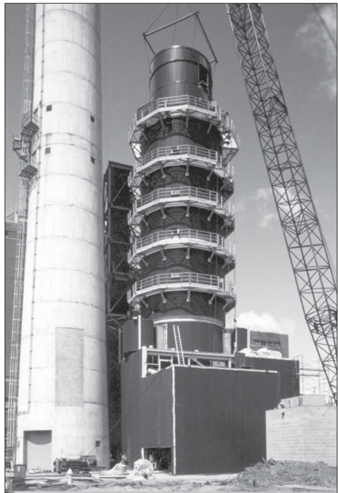
LIFAC activation reactor
