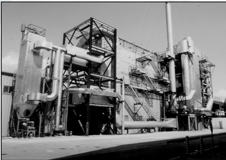
Pulsed Jet Baghouse (left), ESP (center), and GSA System (right)
