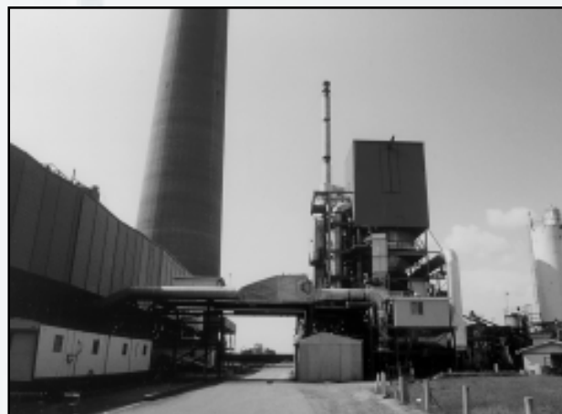
Flue gas slipstream ductwork
