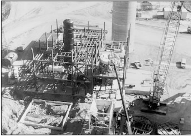
Construction shot with coal screen in foreground, quench table immediately behind, and CDL quench column in the middle
