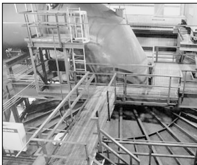
Hot gas duct at top of pyrolyzer
