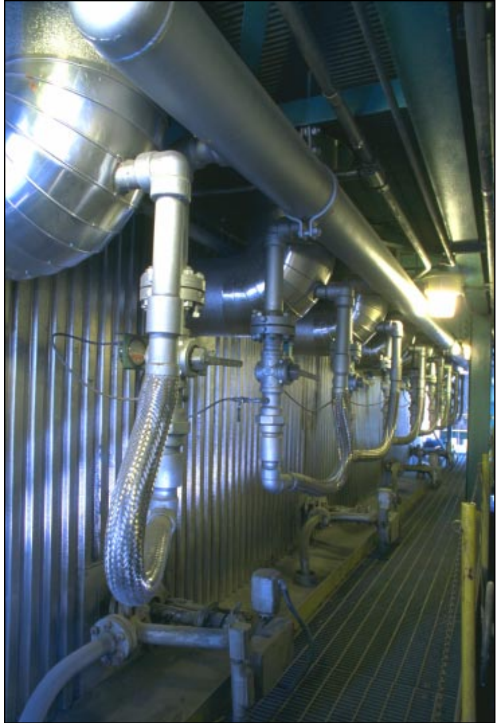
Gas reburn installation on Cherokee Unit 3.
