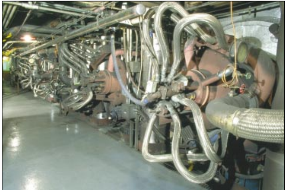
View of low-NO x burners after installation.
