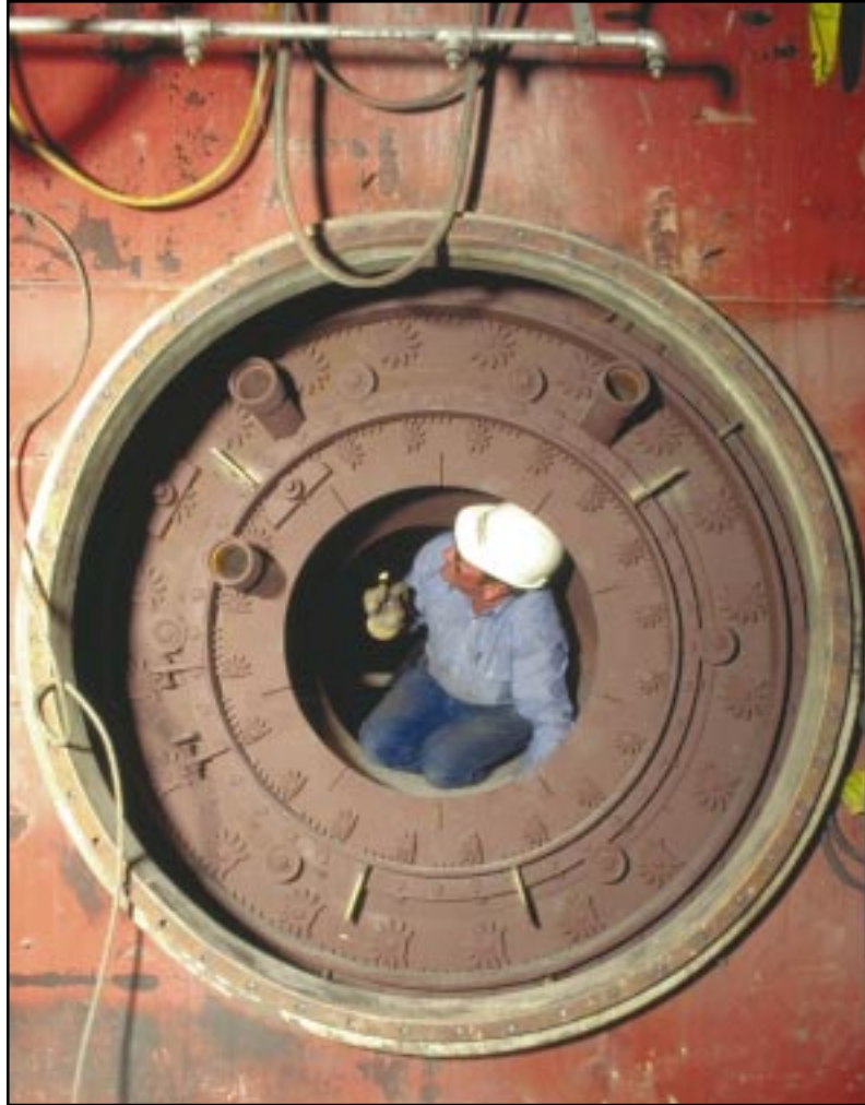
Installation of low-NO x burner.
