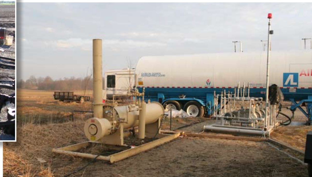
CO 2 storage tank, inline header, and pump equipment at EOR I site.
