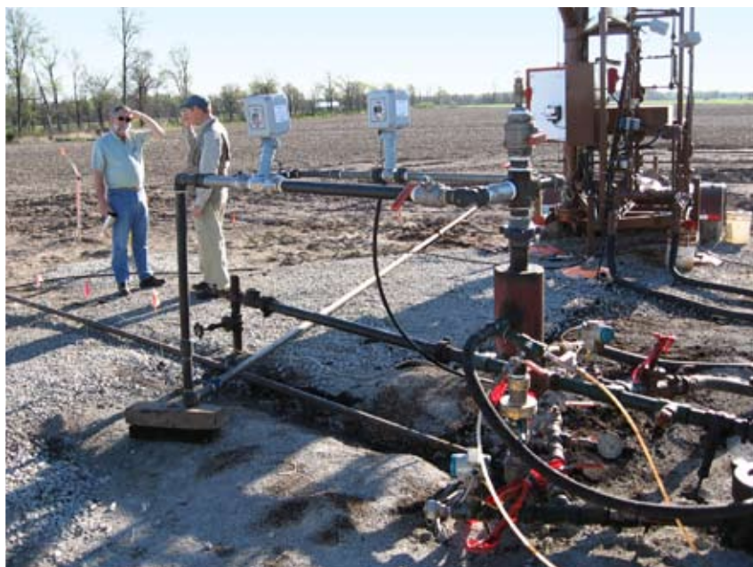
Casing gas production manifold and portable separator at EOR I site.
