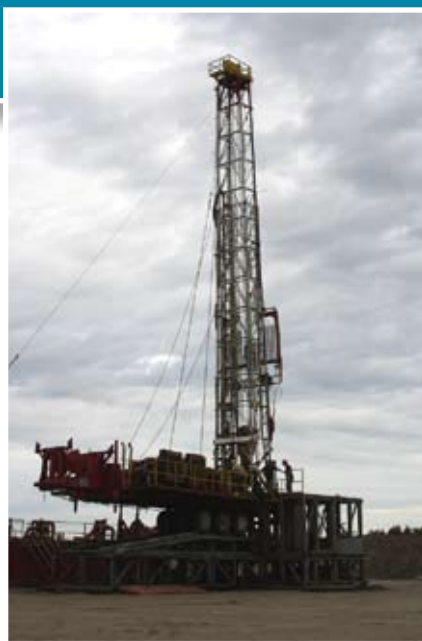
Drilling operations at Mississippi Power's Plant Daniel. Courtesy of Southern Company and ARI.
