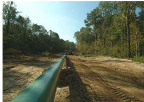
Pipeline (Source: Denbury Resources).
