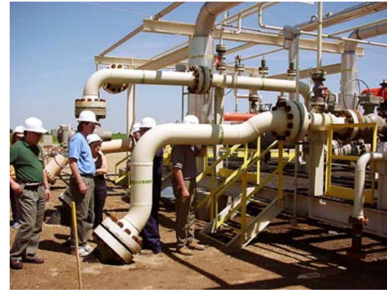
Photo of point where CO 2 exits the underground pipeline that transports CO 2 from Beulah, ND to Weyburn, Saskatchewan (photo courtesy of PTRC and the IEA GHG Weyburn CO 2 Monitoring and Storage Project)
