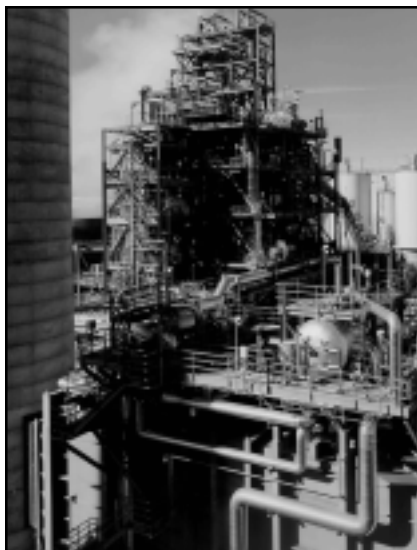
The KRW gasifier island located at the Piñon Pine IGCC Project.
