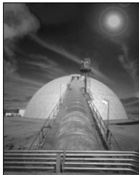
The coal conveyor moves coal to the Piñon Pine storage dome.
