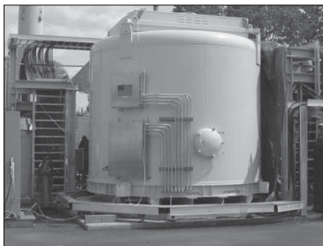
1-MW DFC fuel cell module
