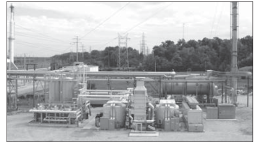
World's largest clean coal-powered fuel cell power plant installed at WREL
