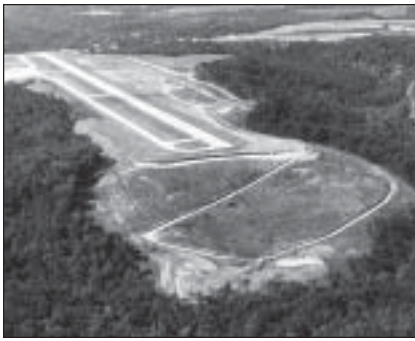
Rostraver Airport near Pittsburgh, Pennsylvania, with CUB project safety area in the foreground
