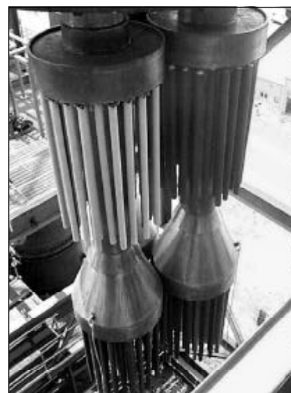
Candle filter arrays for the Siemens Westinghouse hot gas filter system at the PSDF in Wilsonville, Alabama.
