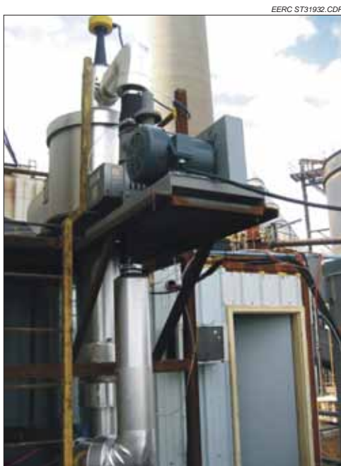
Powerspan ECO slipstream reactor installed at MRYI during testing by the EERC
